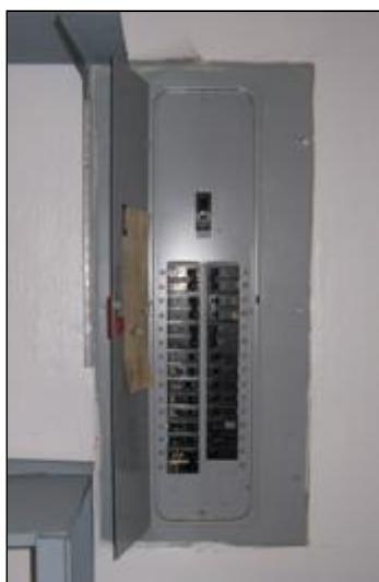
7.6 Picture 1 Main Panel
